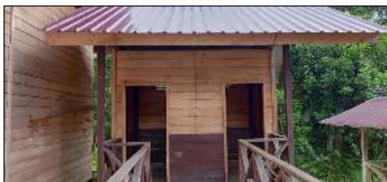
Gambar 4.62. Water Closet SDN 004 Long Isun
