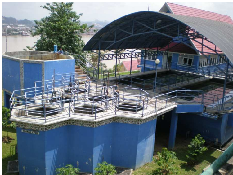
Lampiran 7.10 Instalasi Pengolahan Air (IPA) Gn. Lipan PDAM
