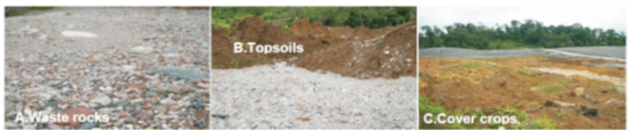
Fig. 2. Initial condition of minedout forest land : A. land preparation layered waste rocks, B. Topsoils spreading, and C. Planting cover crops (2006)
