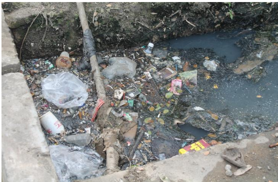
Figure 2. Piles of garbage in Waterways
