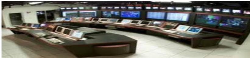
Gambar 4.13. Master Control Room
